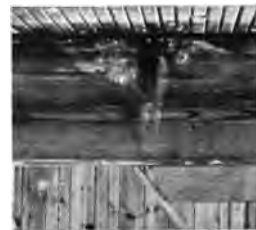
Fig. 4.* (a) Section of bored pine column, affected by dry rot. (b) Fungus growing between double beams, front beam having been removed.
